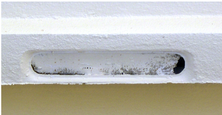
Figure 10. Paint easily bridged the gaps in this \frac{1}{16} -inch mesh screen, reducing the effectiveness of this vent to allow air flow. Note that the screen has become detached from the substrate on the right-hand side. Embers could easily enter through this gap. Photo: Stephen L. Quarles.
